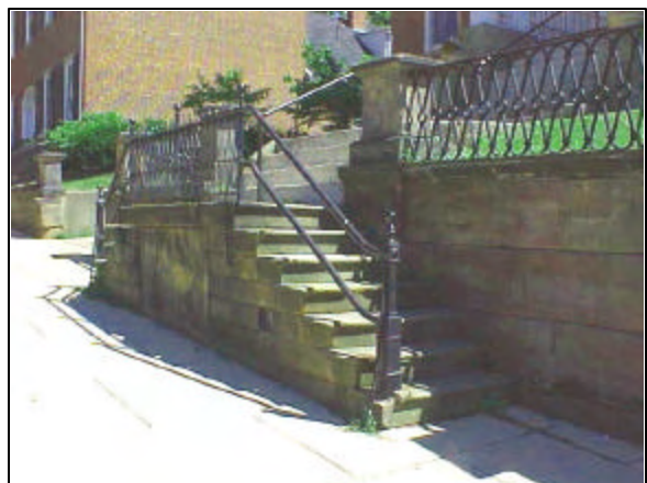
{Photo 2} Local sandstone blocks and slabs form retaining wall and steps. This is a common Lancaster feature.
