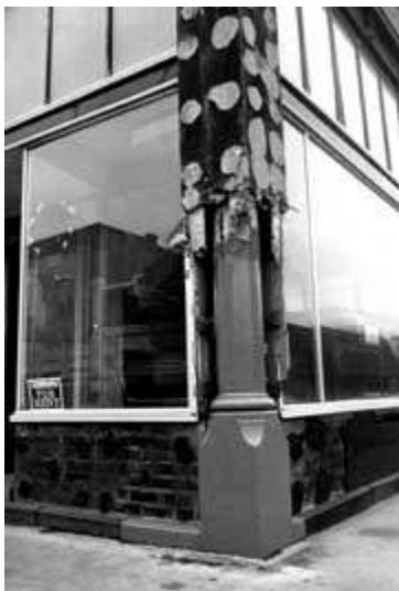
Storefronts of the 1940s, 50s, and 60s were frequently installed by attaching studs or a metal grid over an early front and applying new covering materials. Photo: Bob Dunn.
